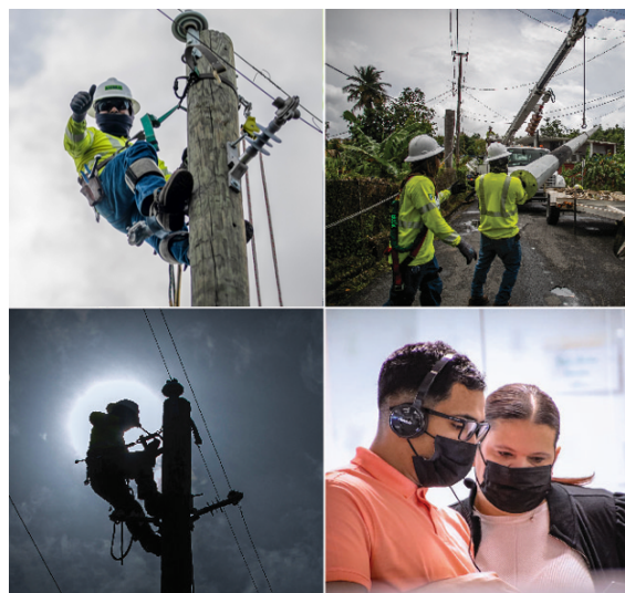
LUMA Energy, Puerto Rico
