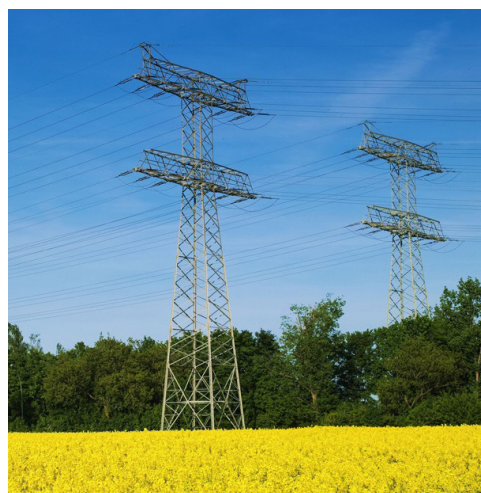
Electricity Transmission Lines
