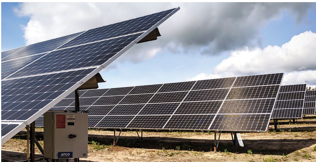
Fort Chipewyan—Canada's largest off-grid solar project.
