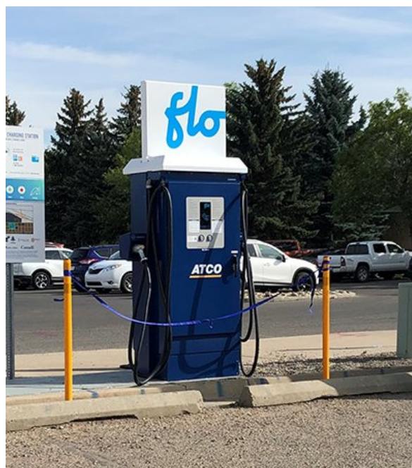
EV charging station, Lethbridge, Alberta
