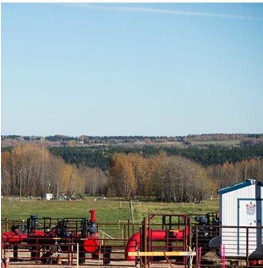
Natural gas transmission control station, Drayton Valley, Alberta
