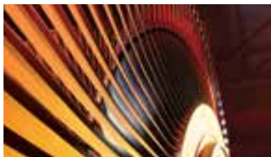
COVER: This turbine is a key component in the process to generate power at the Sheerness generation plant in Hanna, Alberta.
