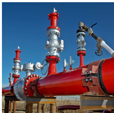
Natural Gas Pipeline Valve Assembly
