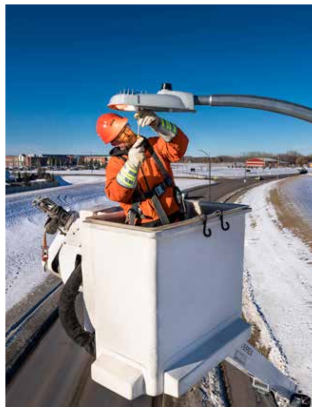
In Lloydminster, we converted outdated street lights to LED bulbs and installed intelligent street lighting sensors. The combined technologies reduce costs, maintenance and greenhouse gas emissions.
