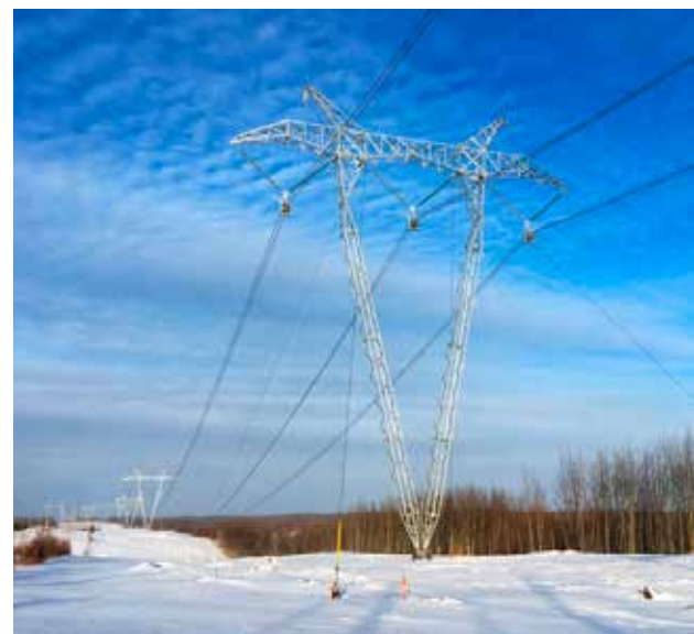
The Fort McMurray West 500-kV Transmission Project, valued at $1.6 billion, was financed in part through the largest public-private-partnership bond in Canadian history.
