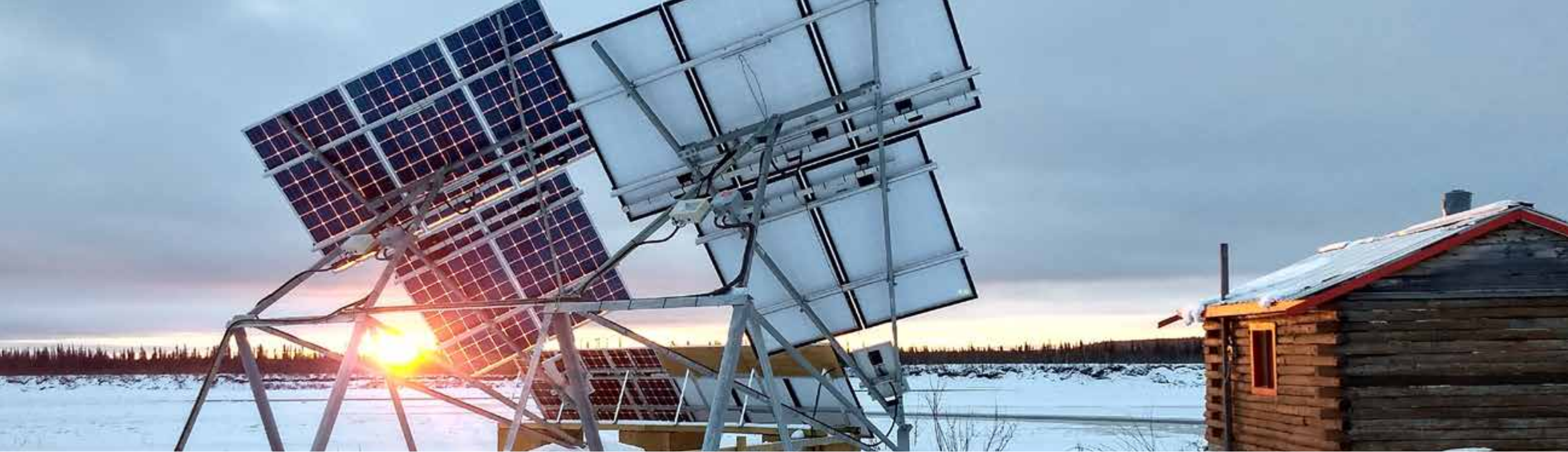
Solar panels, such as these test panels installed at our Old Crow Project site with our Vuntut Gwitchin First Nation partners, help remote communities in Canada's North reduce diesel consumption.
