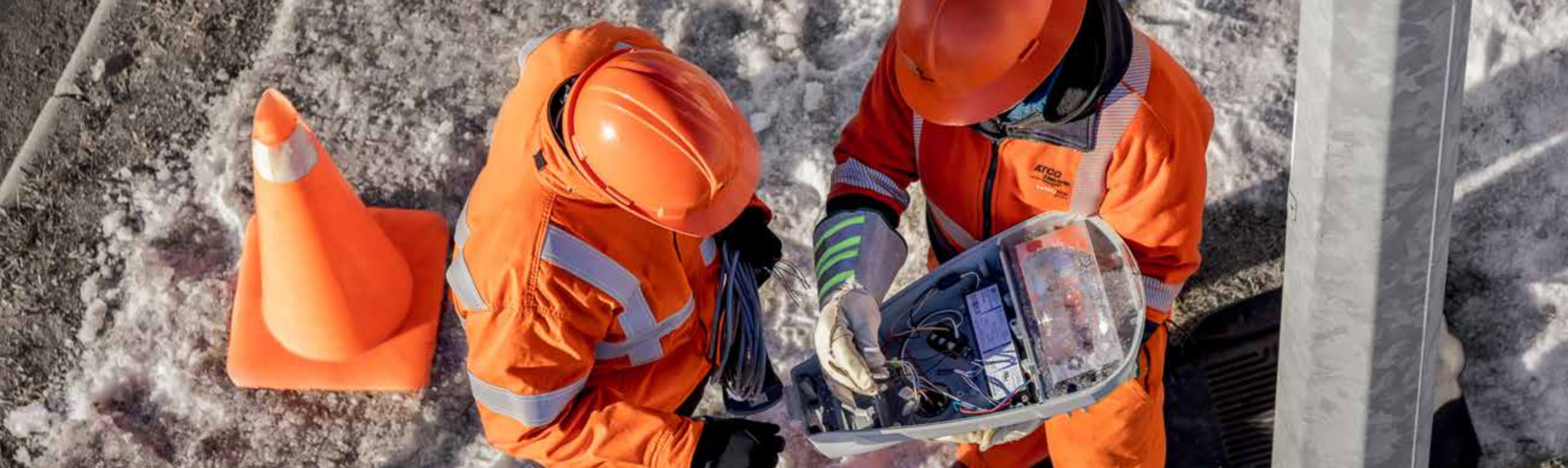
Our Intelligent Street Light Project, in Lloydminster, Alberta, uses wireless motion sensors and a control system for LED street lights to deliver light on demand.
