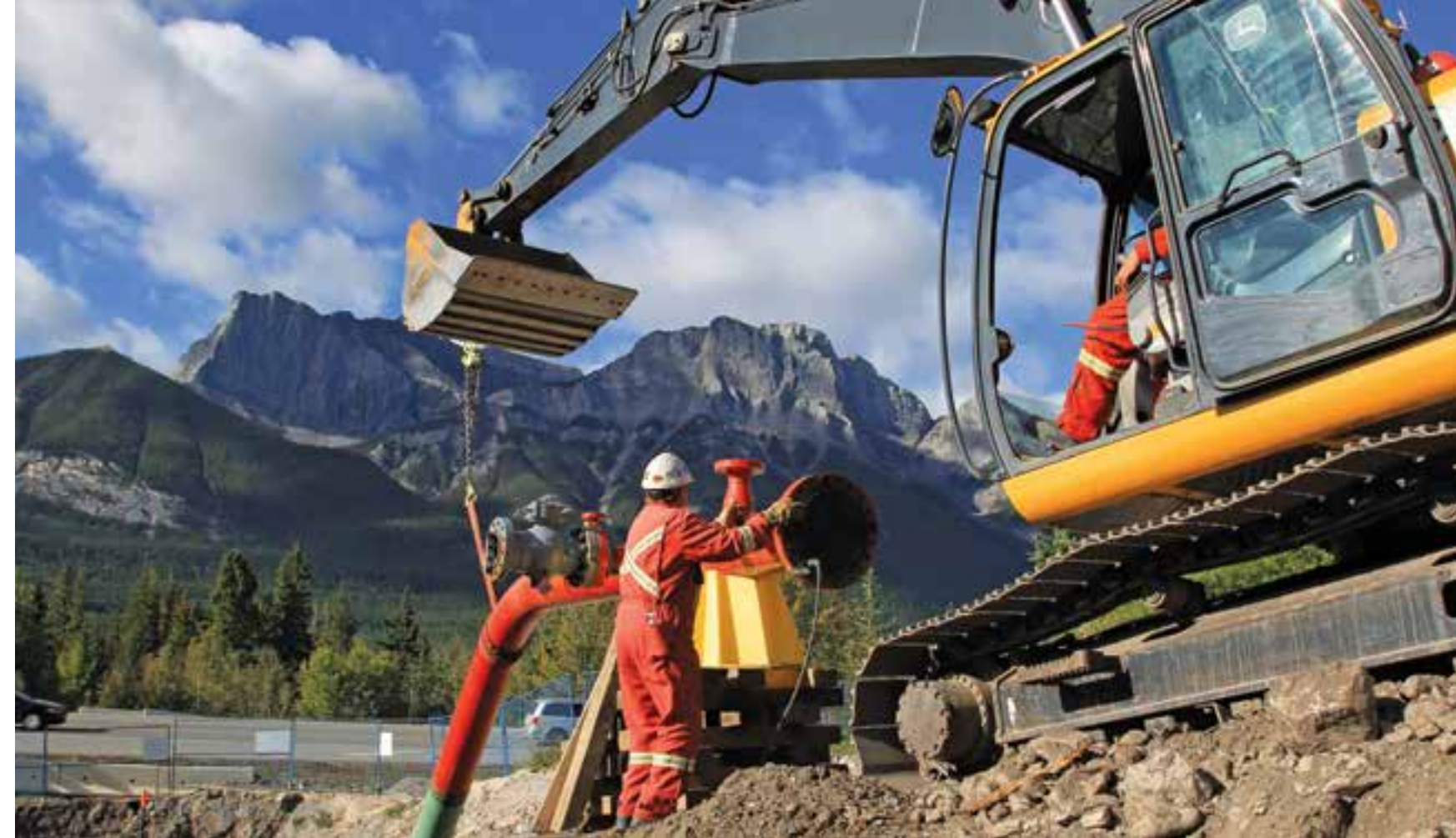
ATCO enabled a key customer in Canmore, Alberta, to use natural gas in place of propane—a safer, cleaner, and more affordable energy source.
