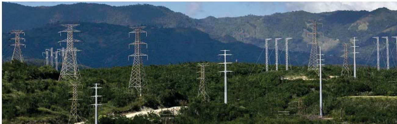
Transmission towers near the Central Costa Sur power plant, Guayanilla, Puerto Rico
