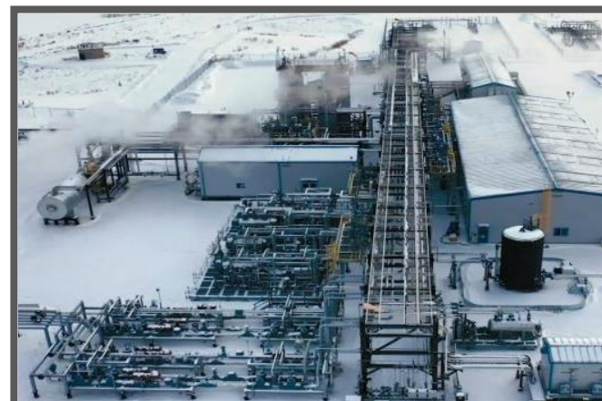
HYDROCARBON STORAGE CANADA 400,000 m 3
